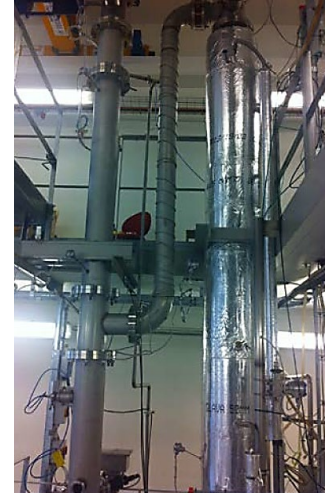
RTI Emissions control (2018-2021) Effective emissions mitigation strategy for WLS at engineering-scale
