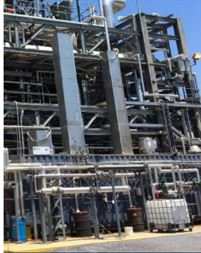
NCCC Pilot Testing at SSTU (2018) Degradation, emission, and corrosion characterizations with real flue gas
