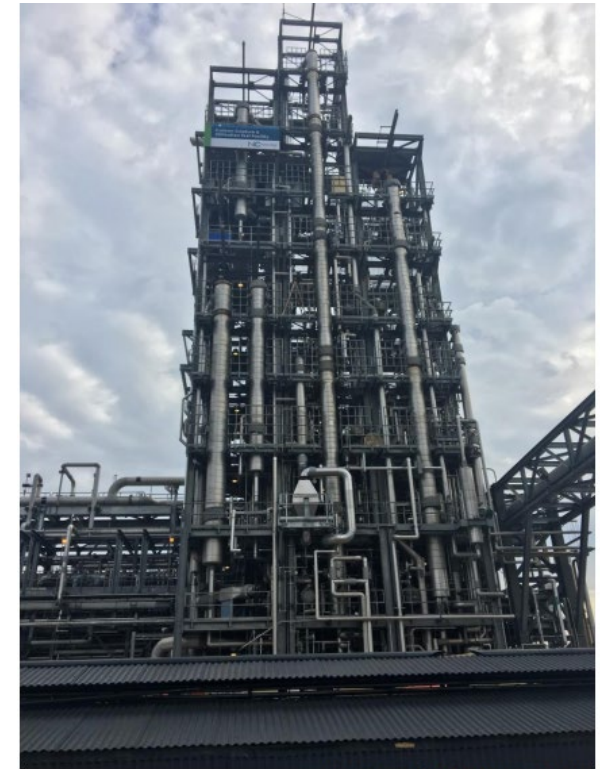
Image courtesy of Southern Company Services PSDF at NCCC
